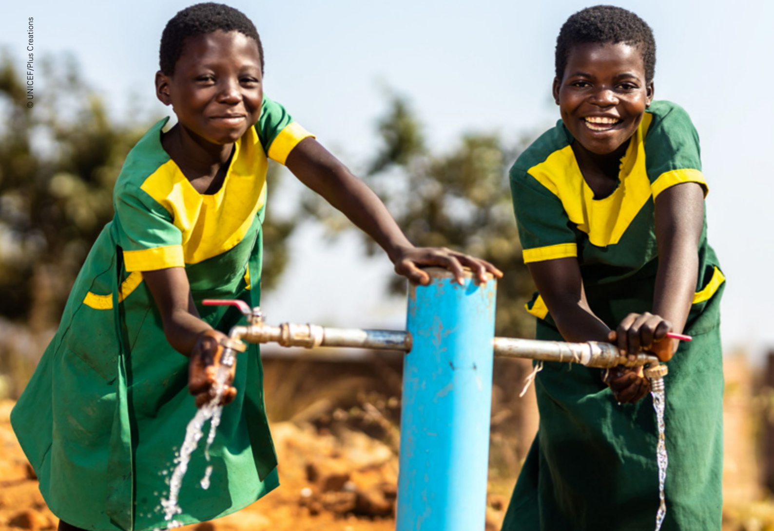
Above: Thokozani Aliko, age 11, and Joyce Peter, 13, draw safe water from a solar-powered water pump at Chitole Primary School, Malawi.
